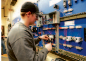
Jonathon Aurand of Selinsgrove wires a reversing motor control circuit in the Electrical Systems Technology program at SUN Tech.
